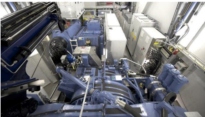
Drivetrain inside the hub of a wind energy system
